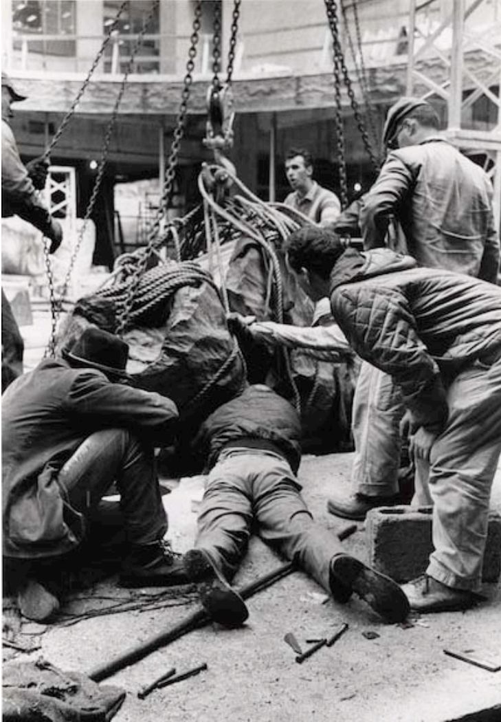
Noguchi (prone) installing a stone for Sunken Garden , Chase Manhattan Bank Plaza, NYC, c. 1964, Photograph: Arthur Lavine
